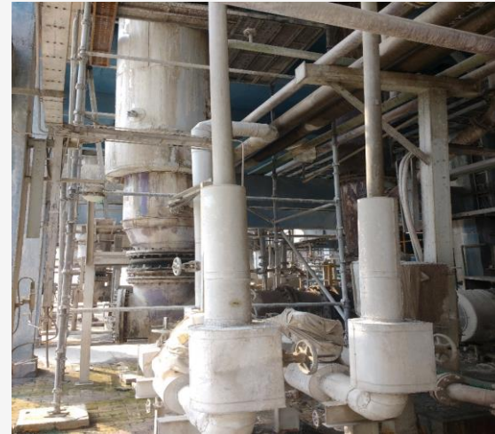
Control valves for condensate export and drain lines
