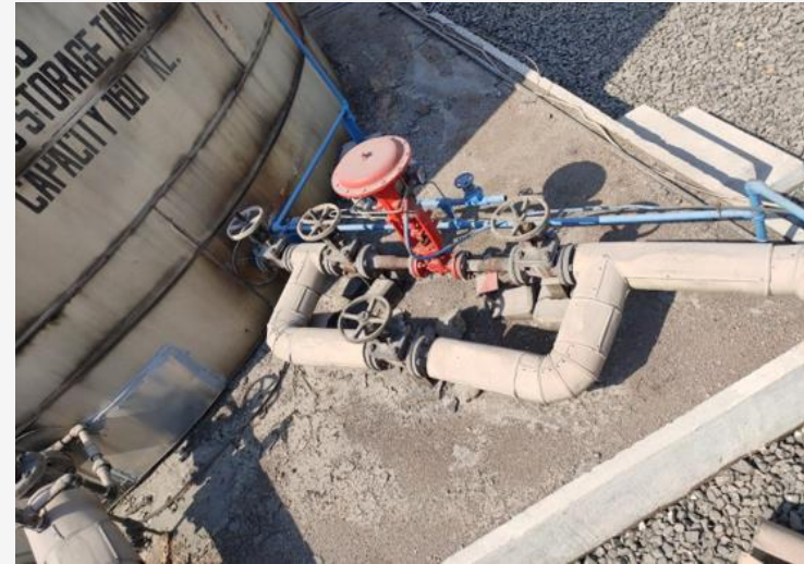
LSHS Tank Fuel Oil Temperature Control Valve
